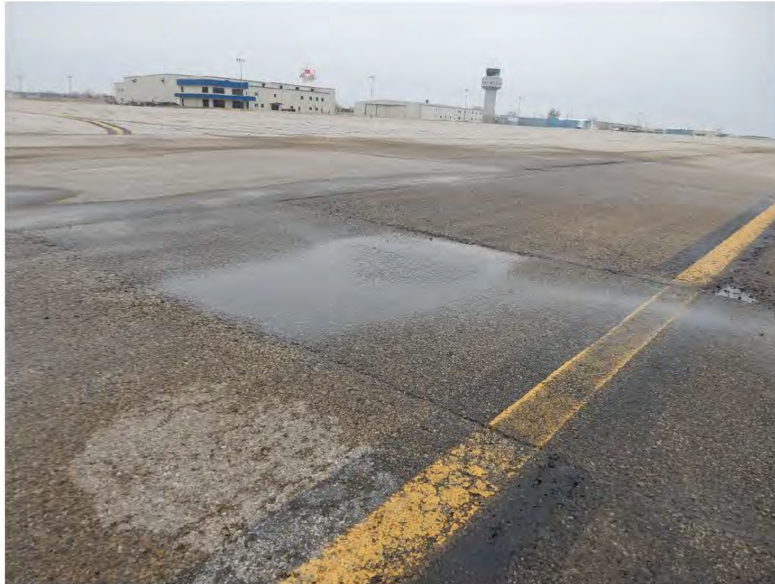
Taxiway Alpha - Ponding
